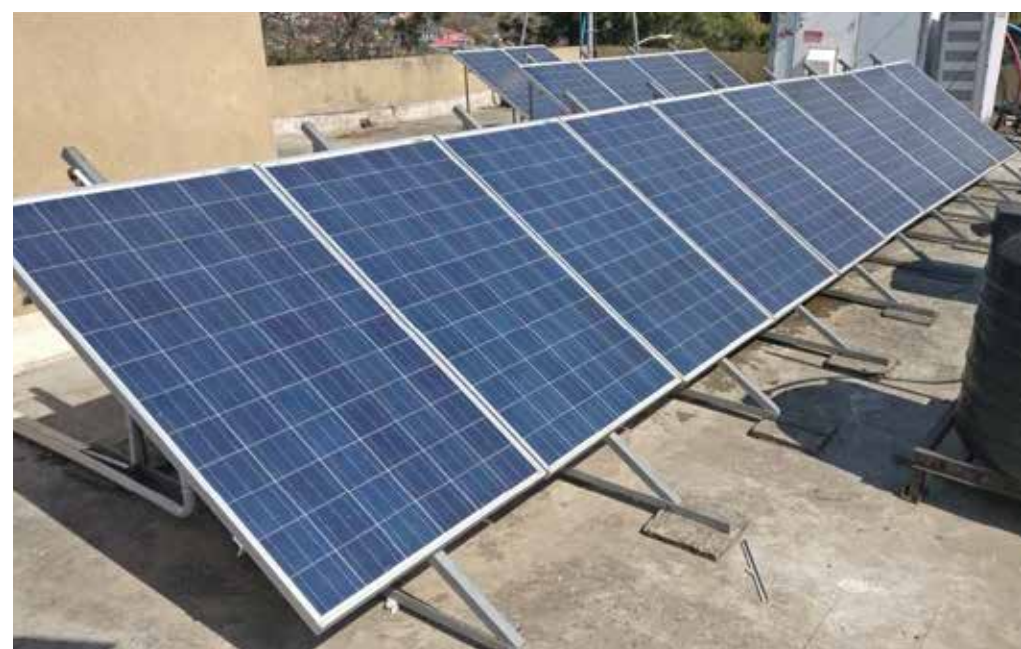
Figure-6: Solar PV module on the rooftop of Municipal Corporation building of Dharamshala Source: Rooftop Solar detailed project report
