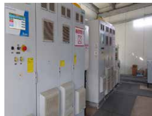
Plate 7. Inverter Rooms converting DC power from Solar Panels to AC, with real time monitoring
