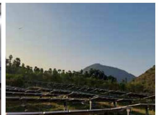
Plate 8. Land based smart solar panels that change directions as per sun path, maintained by GVSCCL
