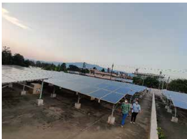
Plate 9. Rooftop Panels over Water Reservoir in Visakhapatnam
