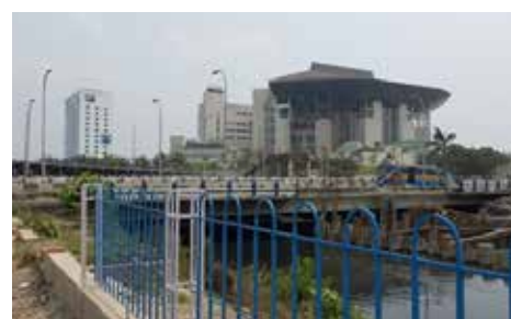
Fig. 2. View of the entire site showing the (a) installed 500 kW unit near Biswa Bangla Convention Centre and (b) civil work for the other 500kW unit on Bagjola canal (Source: Author)
