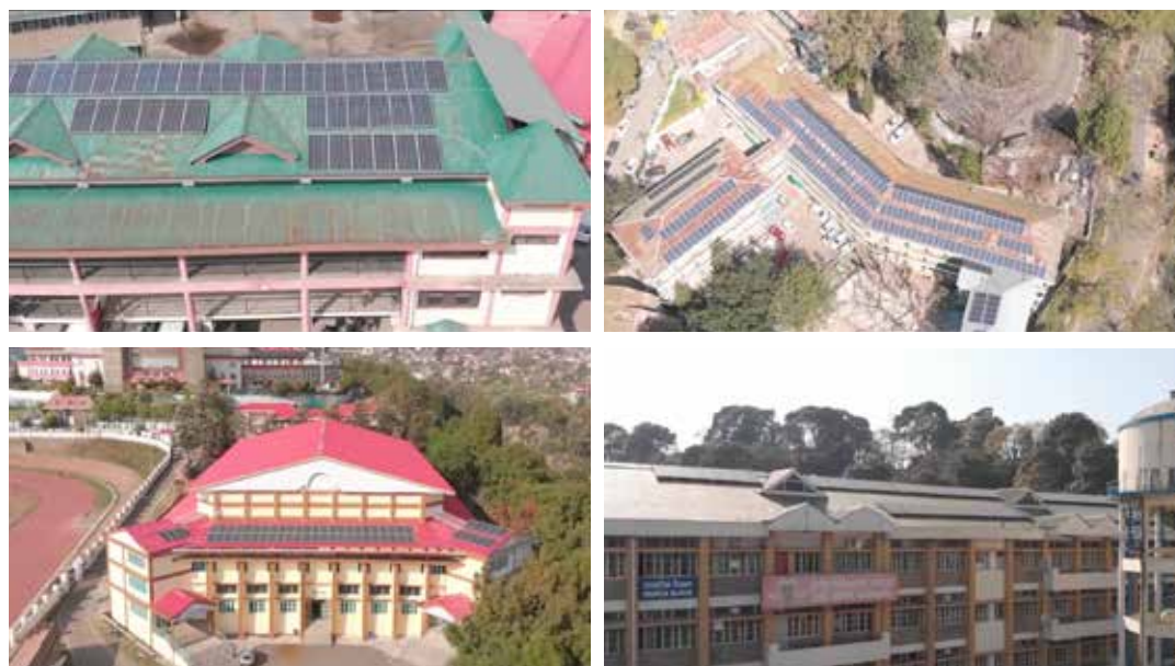
Figure 13. Solar PV system installed on buildings in phase I Source: Dharamshala Smart CitySource: Rooftop Solar detailed project report
